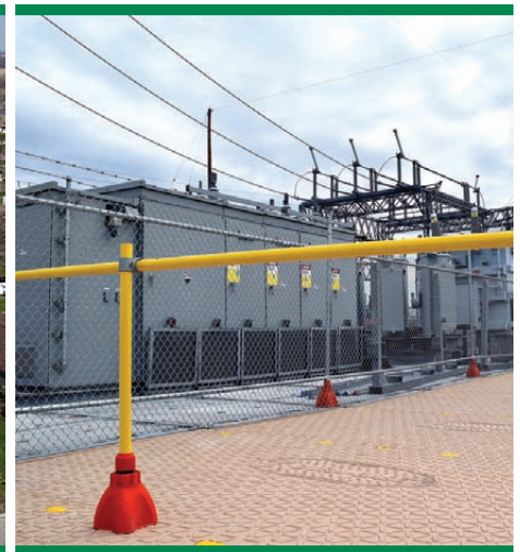
Safety Barrier Fencing Around Substation Project
