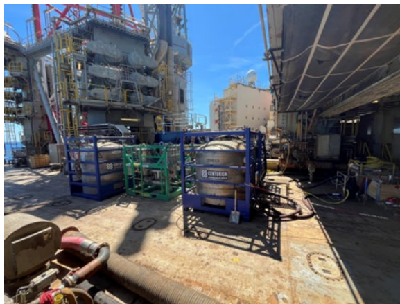
Figure 1 - Fluids Management Package, equipment installed on main deck
